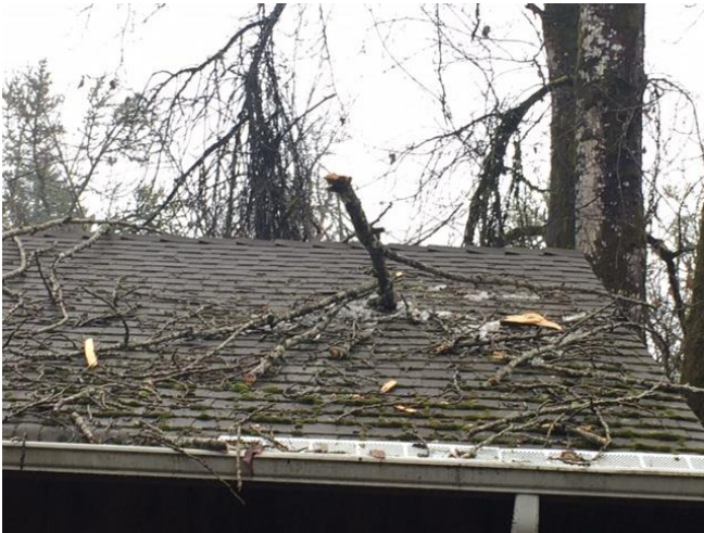
Arboretum center roof pierced
